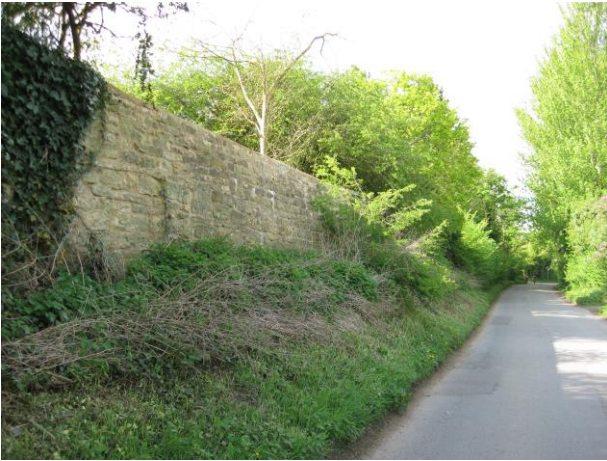
The tall stone wall of Beckford Hall which contributes to the character of the conservation area.
