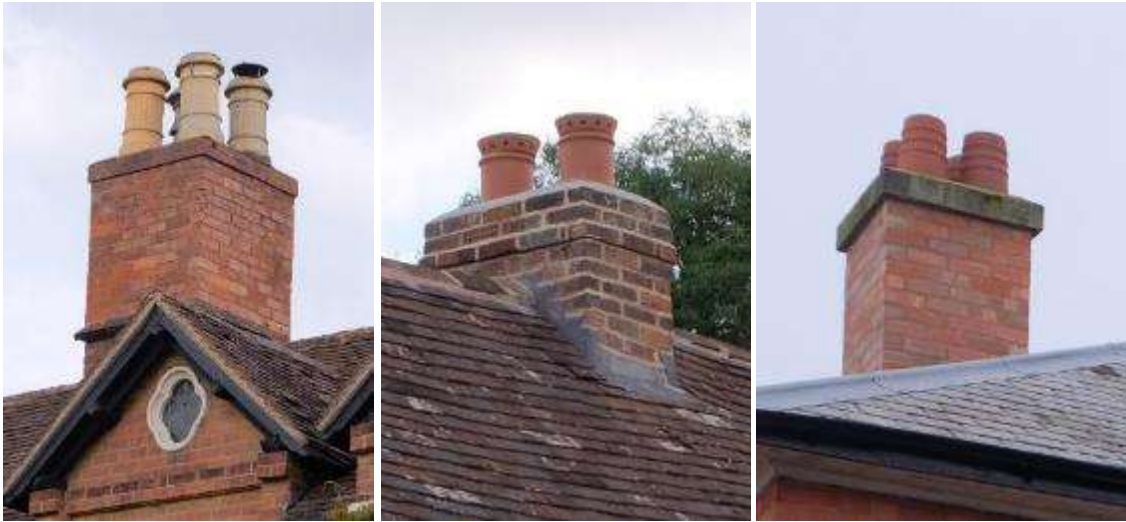
Simple yet robust brick chimneys in Ombersley (left and centre) and Droitwich Spa (right)
