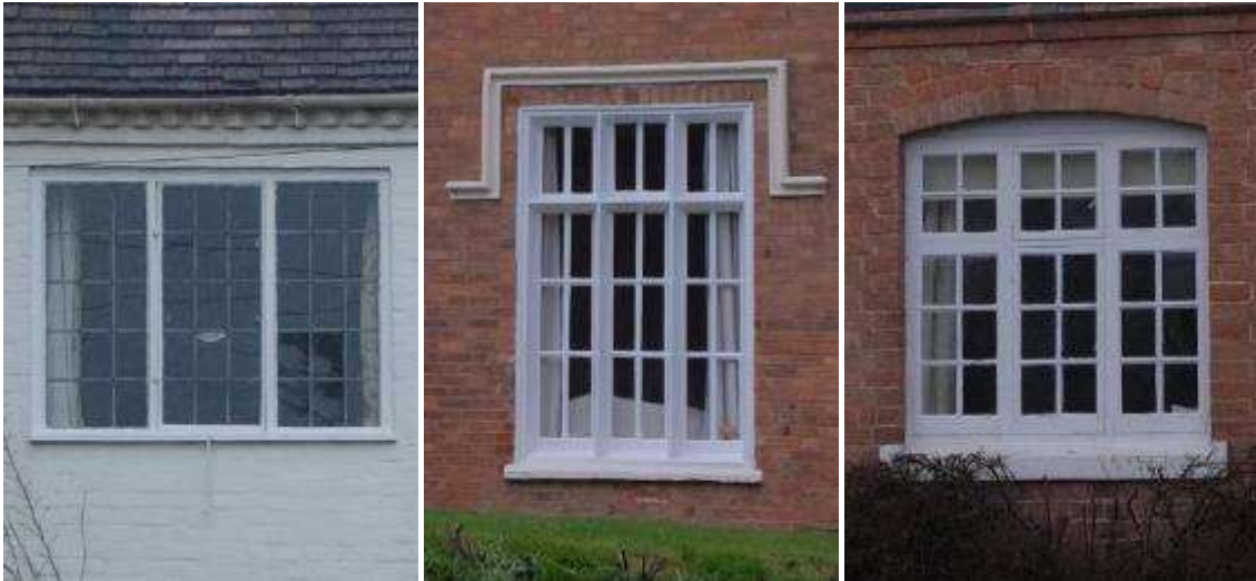
In Inkberrow, 8 pane fixed windows with a central casement (left) and with a transom and mullions (centre and right)
