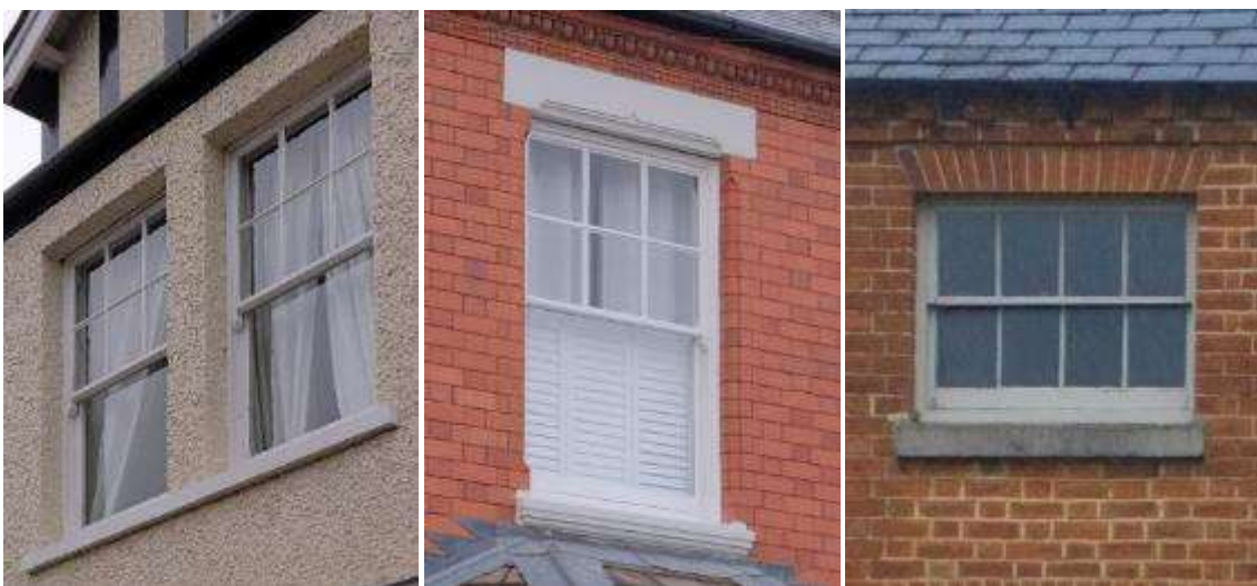
6-over-1 sash windows (left and centre) in Droitwich Spa and a 4-over-4 window in Inkberrow (right)
