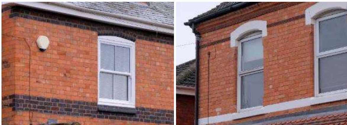
Burnt brick banding (left) and white banding with a brick string course (right) in Droitwich Spa
