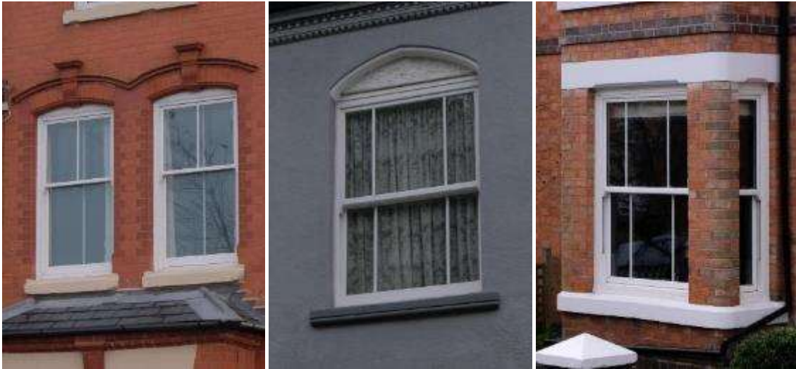
Large 2-over-2 (left) and 3-over-3 sash windows (centre and right) in Droitwich Spa
