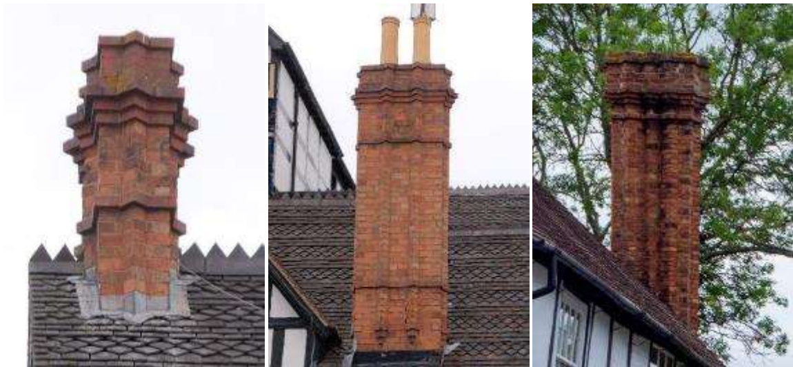
In Droitwich Spa, chimneys with ornamented corbels (left and centre) and in Ombersley (right)
