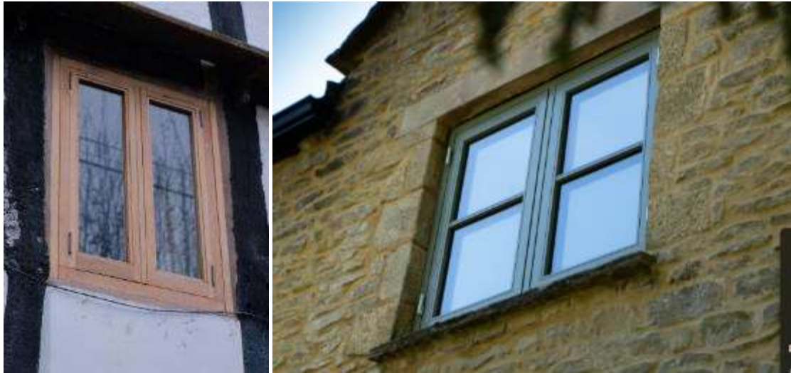
New timber casement windows in Uphampton (left) and timber/aluminium composite casement windows (right, image credit Enlightened Windows)
