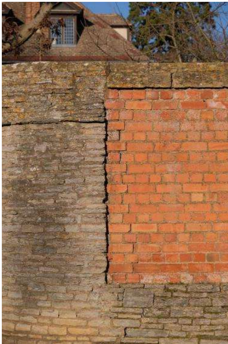
A wall which has been added onto over many years, a combination of various sizes of lias stones with an English bond brick wall
