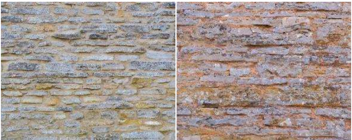
Lias stone walls in North Littleton with irregularly shaped and sized stones
