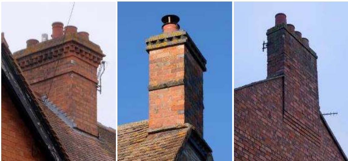
Brick chimney with dentil details in Bretforton (left) and North Littleton (centre) and a gable-ended chimney in Evesham (right)
