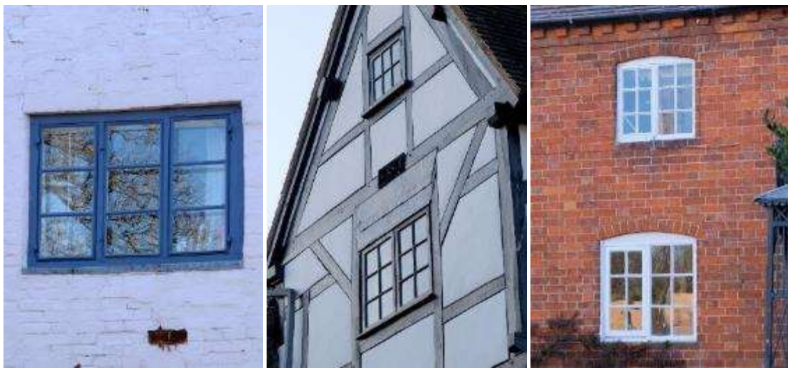
3 and 6 pane casement windows in Pebworth (left), Harvington (centre) and Honeybourne (right)
