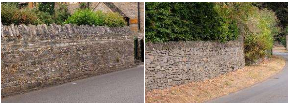
Lias stone boundary walls in Bretforton (left) and Cleeve Prior (right), the latter with a wide green verge separating the wall from the street
