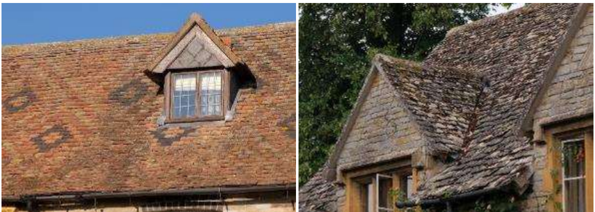
Clay tiles with an ornamental pattern in North Littleton (left) and Cotswold stone slates in Bretforton (right)
