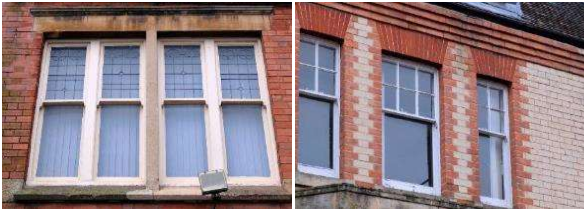
Ornamental sash windows (left) and 4-over-1 and 6-over-1 windows (right) in Evesham
