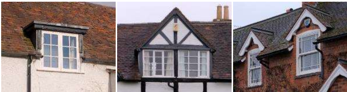
A flat roof dormer in Great Comberton (left) and a large wide dormer window (centre) and wall dormer windows (right), both in Crowle
