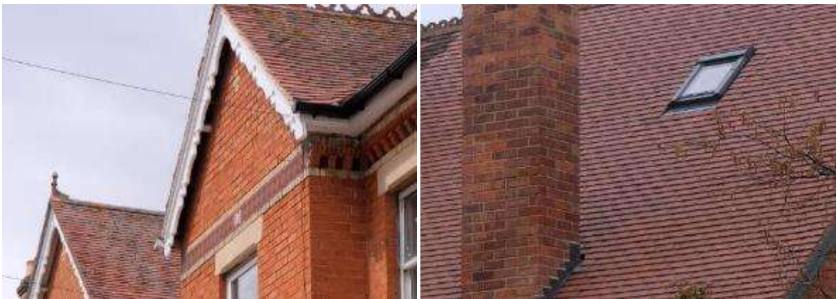
Roof tiles in natural clay in Pershore (left) and imitation clay in Eckington (right)
