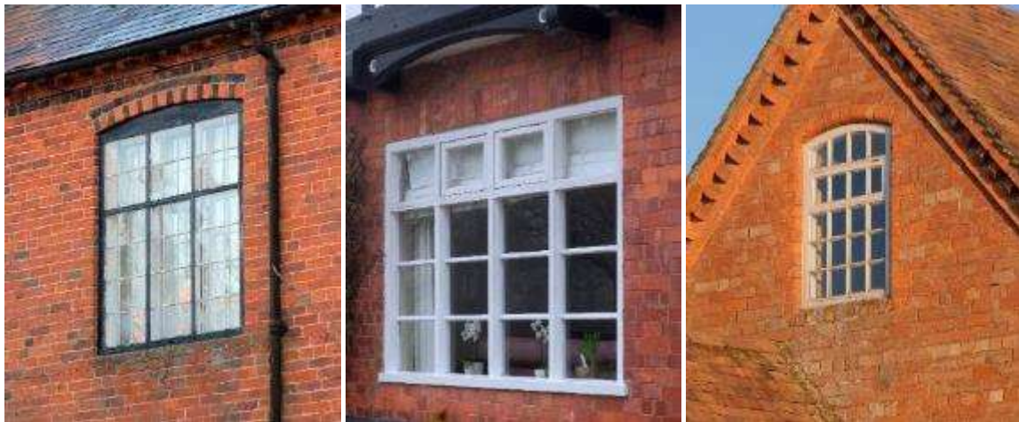
Fixed windows in Atch Lench (left) and windows with small top-hung fanlights in Rous Lench (centre) and Atch Lench (right)
