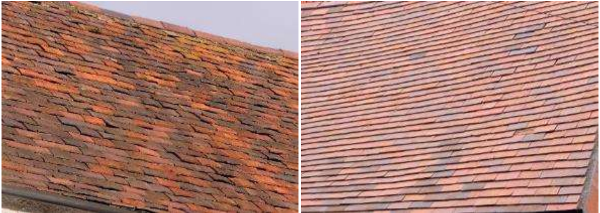
Roof tiles in natural clay in Great Comberton (left) and imitation clay in Fladbury (right)
