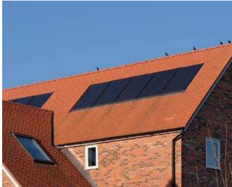
Solar panels integrated flush with the roof on a house in South Littleton
