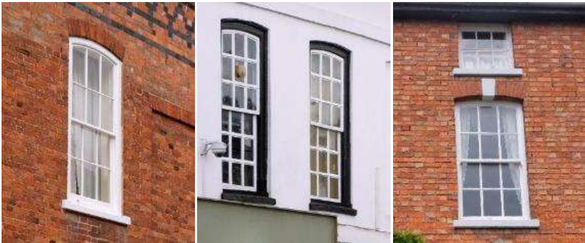
Arched 6-over-6 sash windows with white and black and white frames in Fladbury (left) and Pershore (centre and right)
