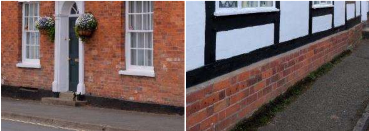
A painted plinth in Persore (left) and a brick plinth on a timber frame building in Church Lench (right)
