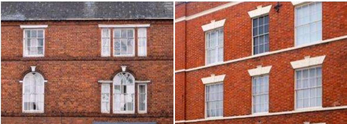
String courses in matching brick (left) and contrasting colour (right) in Pershore
