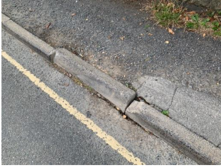
Damage to the foot path caused by heavy vehicles adjacent to the SG chosen Development site
